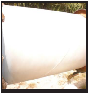
Above: Finished pipeline insulated with Nansulate® Translucent PT Right: Technician applies coating with spray equipment in the field
