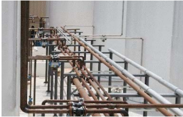
Steam lines insulated with Nansulate® High Heat.
